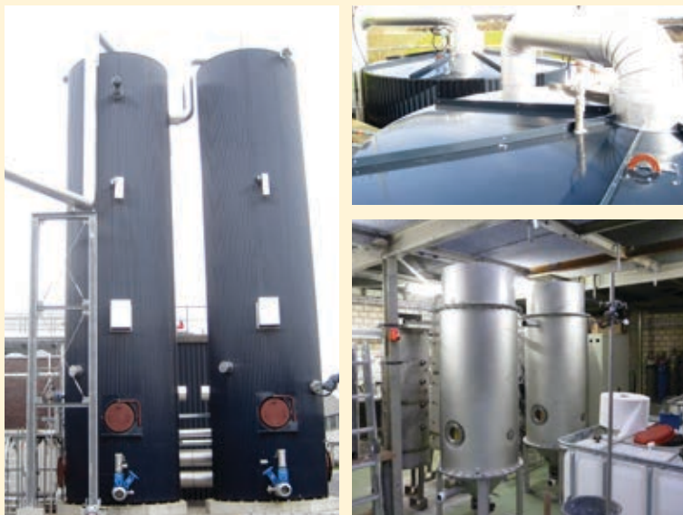
Fig. 5 The two biofilm digesters in Gescher are 12.5 metres high with a 3-metre diameter. Left and top right: Digester in Gescher. Below right: The plant in the laboratory.
