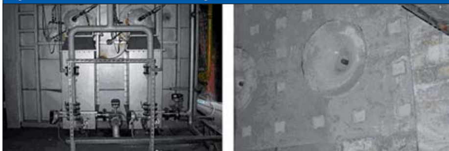
Fig. 3: Flat-flame burner with thermal regenerator
