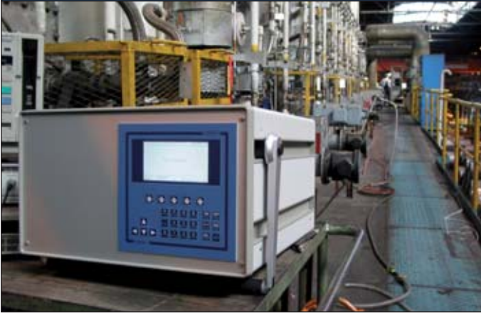
Fig. 5: New measurement system for furnace atmospheres
