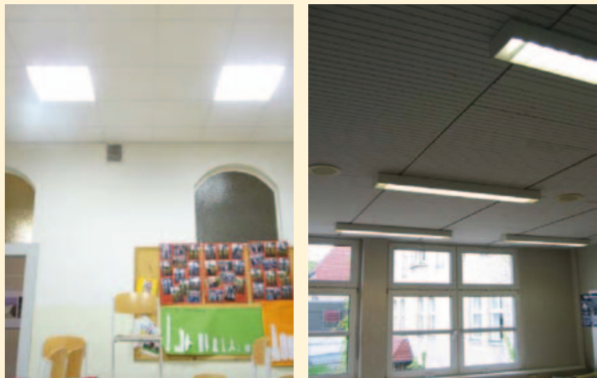
Fig. 1 Typical existing situation with grid luminaires including fluorescent lamps and low-loss ballast devices: Left in the old building, right in the extension. Source: TU Berlin
