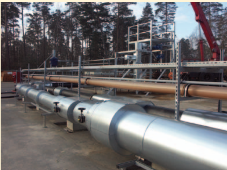
Fig. 4 Corrosion research in a bypass of the thermal water circuit in Groß Schönebeck. Source: German Research Centre for Geosciences in Potsdam
