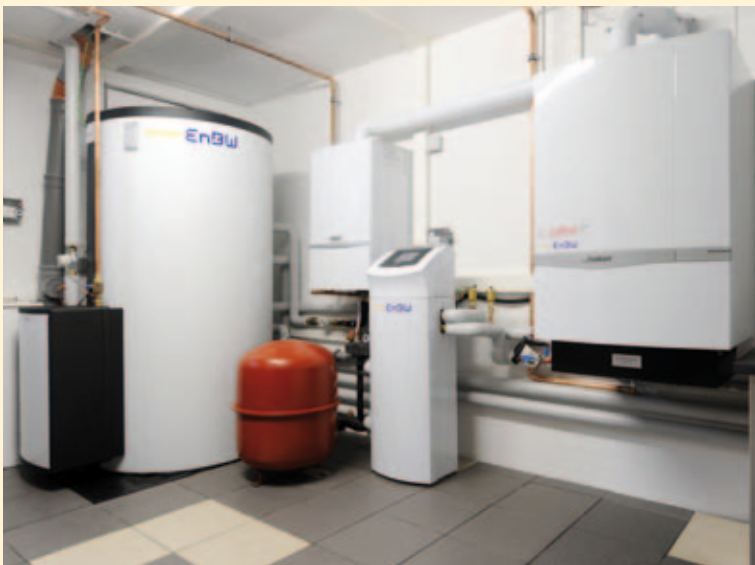
Fig. 4 Fuel cell heating unit in a basement Source: Vaillant GmbH
