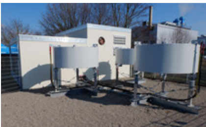
An inductor is connected parallel to the fault current limiter for every phase. © Dr. Franz Meyer, BINE Informationsdienst
