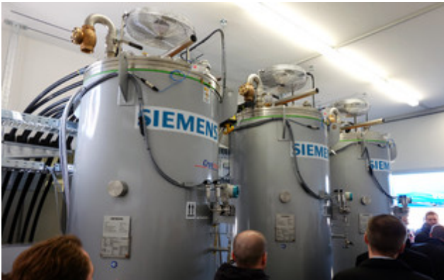
The fault current limiters for the three phases of the electricity grid are housed separately in cryogenic containers. Closed cooling systems ensure the low temperatures. The whole system is so compact that it can be housed in a prefabricated container. © Dr. Franz Meyer, BINE Informationsdienst
