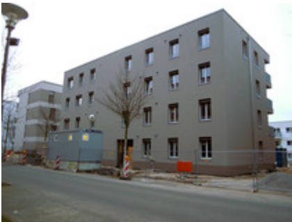
House 2 with a solar thermal energy system and the technical centre during the construction phase.
