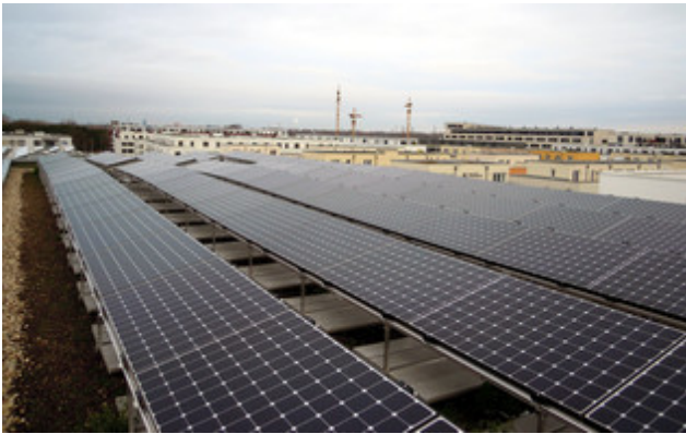
Photovoltaic system on the roof of House 1, one of three four-storey residential buildings that are being constructed during the first construction phase.
