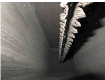
Interior view of the precipitator box: The deposited particulate matter can be seen at the electrodes. © IZES
